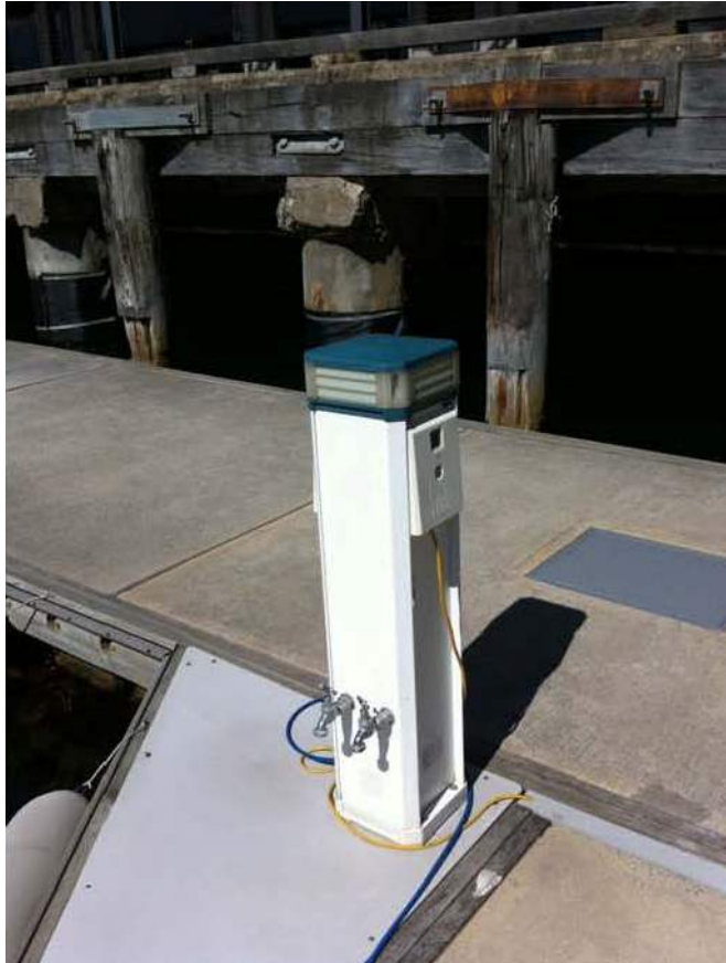
Photograph 2.1 Services pedestal similar to that proposed for Georges Cove Marina (photographed at Jones Bay Wharf in November 2010)
