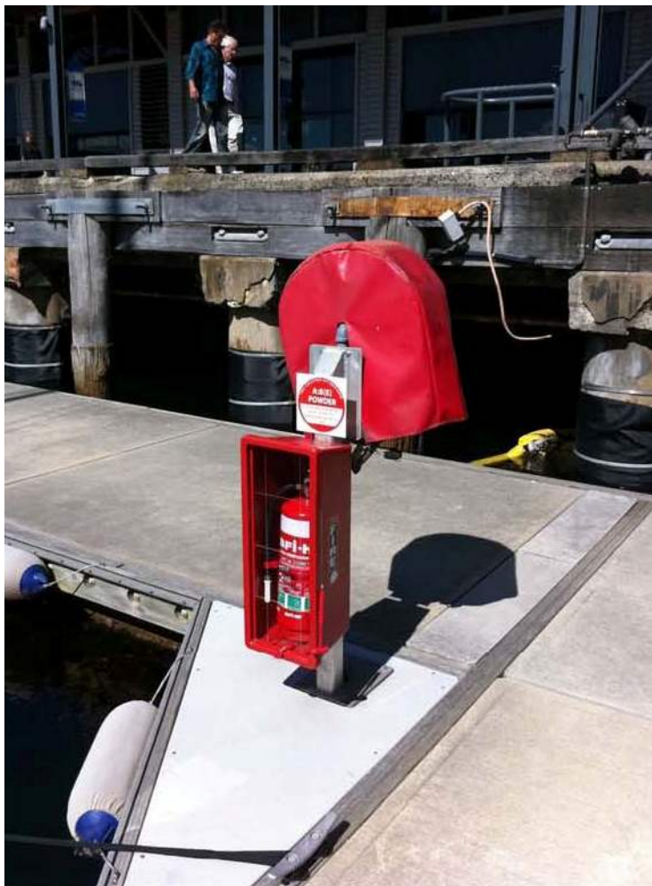
Photograph 2.2 Example fire extinguisher and hose
